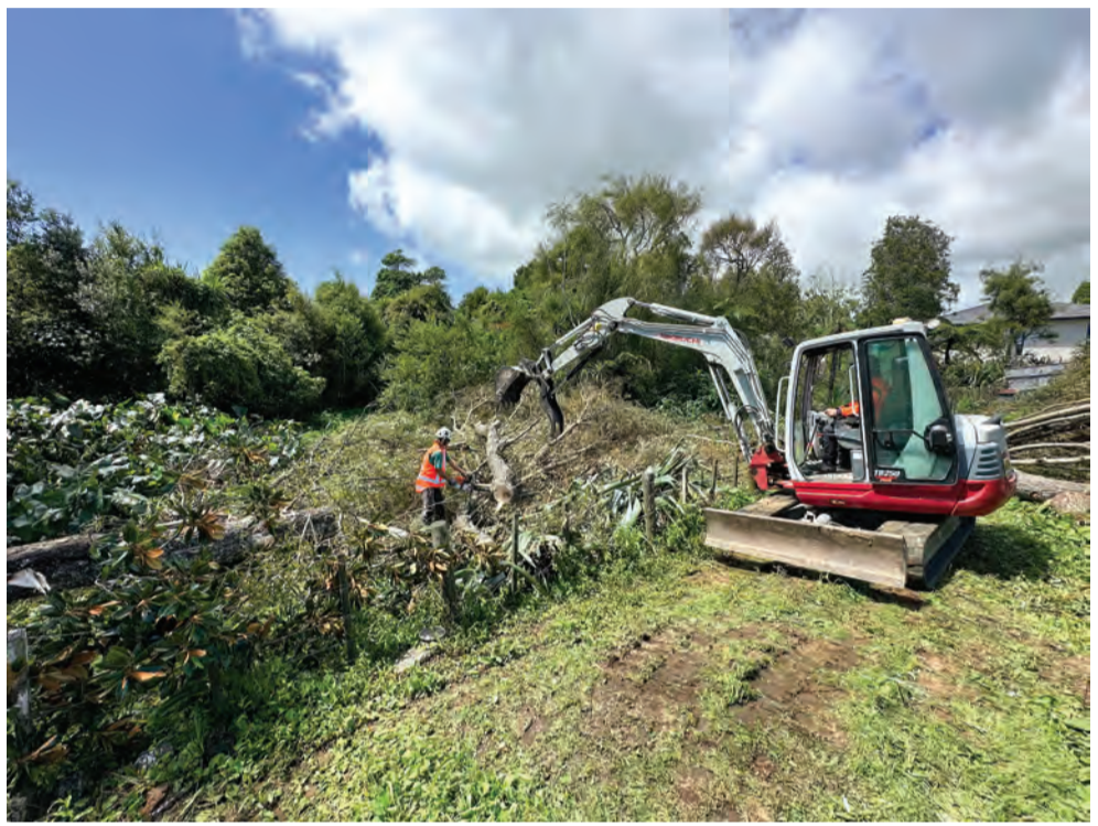
Work is underway to clear trees and invasive weeds from the banks of the Tangaroa Stream.
